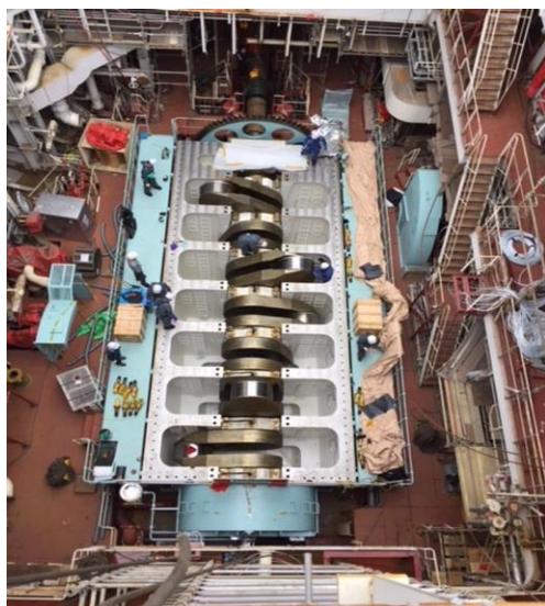
Main engine bedplate with crankshaft installed on the first Aloha class ship.
